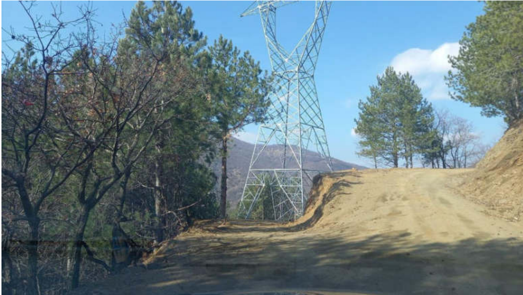
Photo 14-2: Illustration of the area where the MT cable will be routed (2 of 2)
